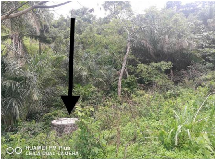
Water reservoir tank in Finge
